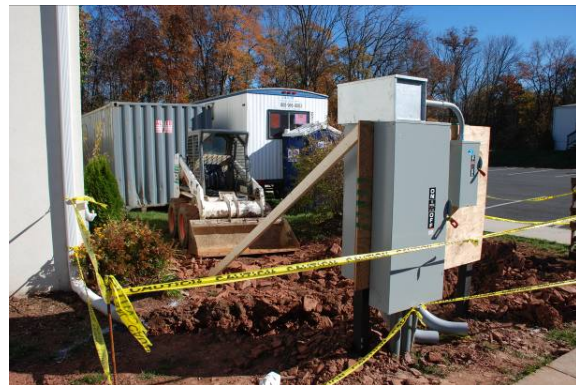
Ready for Temporary Power, November 2010
